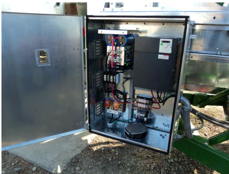
DC Power Supply shield removed to show detail.
